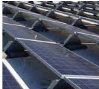
Solar array on roof
